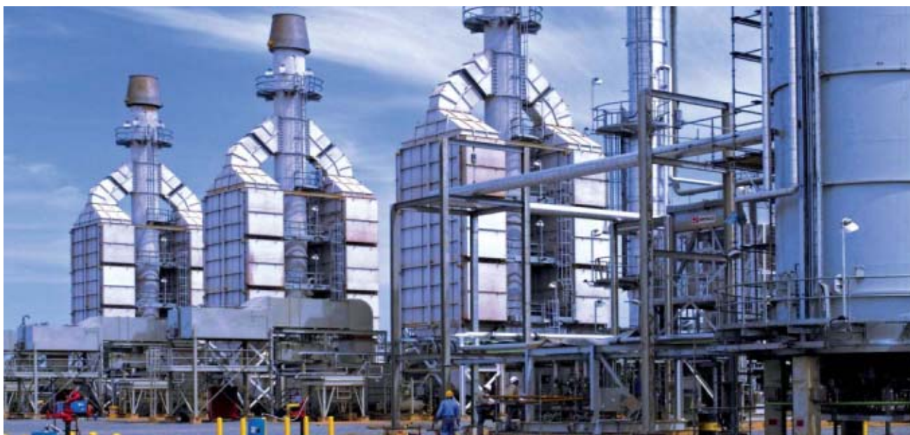
Pump Station, Dompta.
