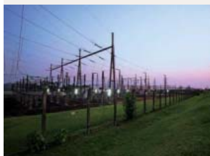
Electricity plant, Logbaba.
