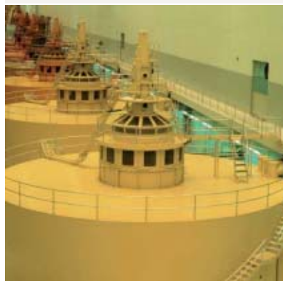
Generators room plant.
