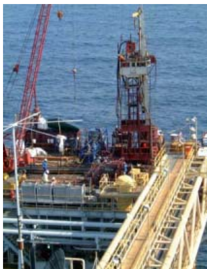
Hydraulic workover unit on Bravo platform.
