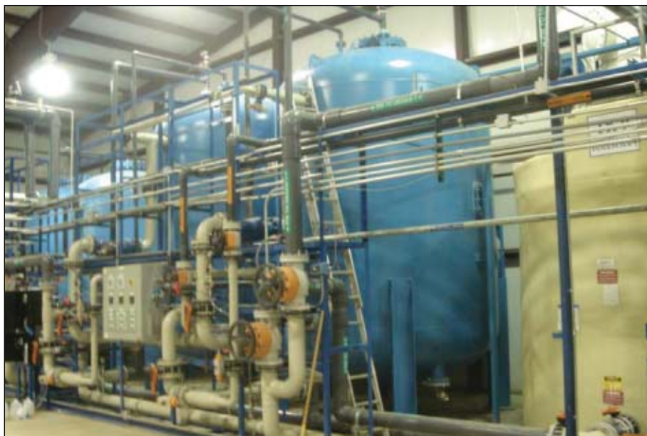
The treatment processes includes three storage tanks for breaking the regeneration cycle into segments (Fig. 2).
